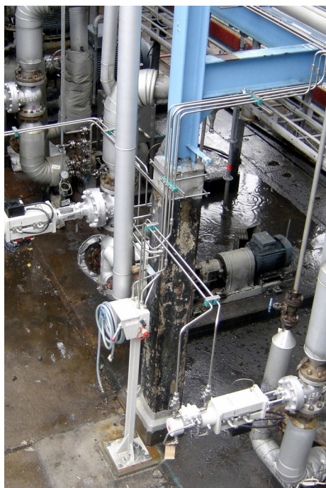
Hydraulic Actuators with gate valves
